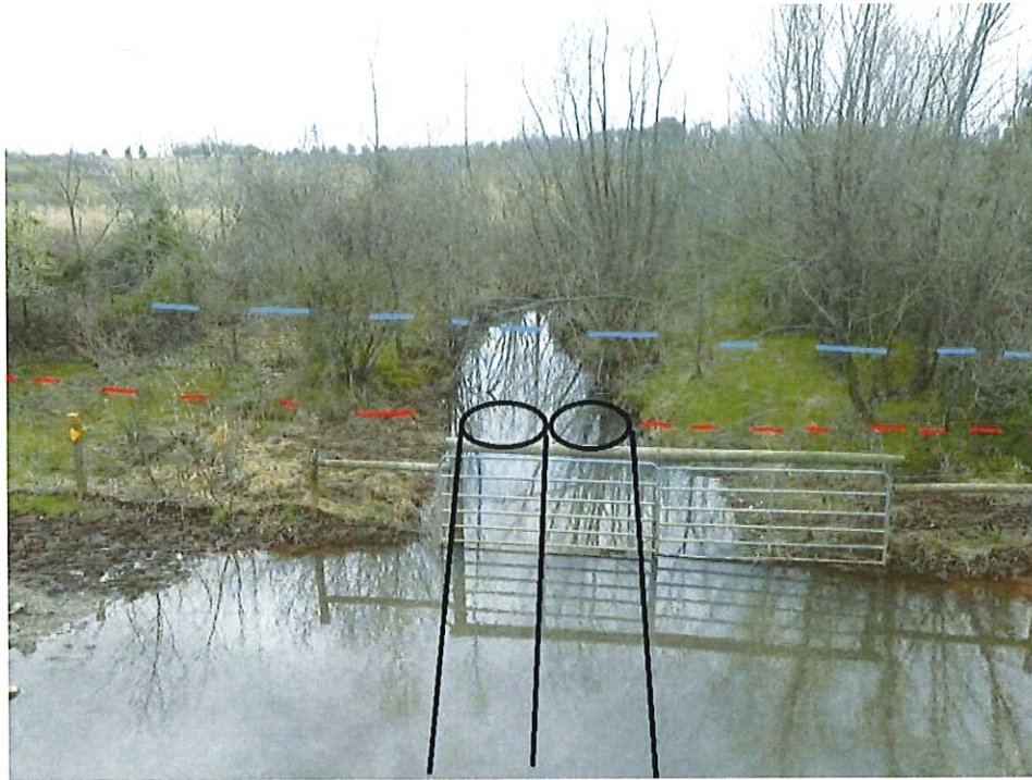
Photo 2.1 Facing south from existing bridge showing approximate edge of take (red-line), temporary easement disturbance (blue-line), and temporary detour culvert locations.
